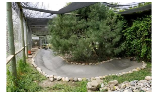
Creek with its coat of sealant rock. We were able to restore the plants, none the worse for wear after we had set them aside when we first began the project.
